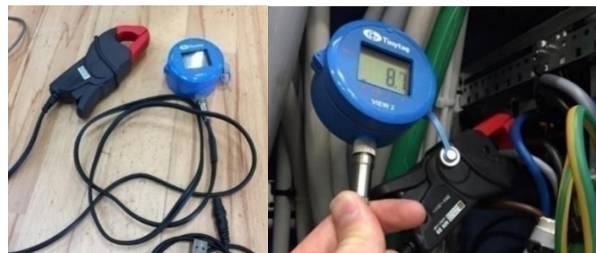
Figure 40: Tiny Tag Data logger with a current clamp.
